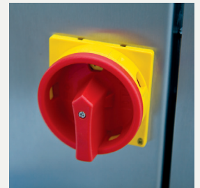
The main circuit breaker
